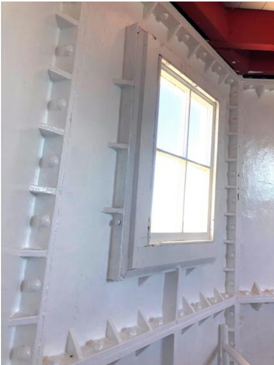
Boulder Bank cast-iron interior
