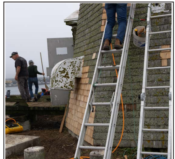
Temporary shingle replacement was required for areas with extensive damage, and for areas where access to the wood below was required.
